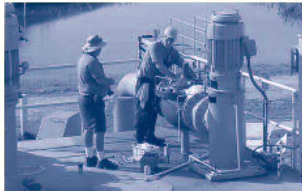
Ron Prue (left), maintenance technician at Peace River Facility, and an employee from Bob Dean Supply work to repair a transfer pump.
