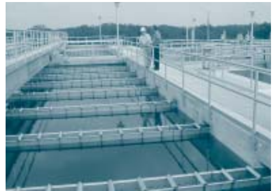
Pat Leberman, executive director of the Authority, and Doug Eckmann, project manager for Boyle Engineering, inspect the expanded plant. The December 1, 2001 target operational deadline was met.
